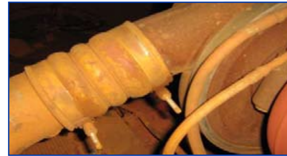
Figure 5: Example of the hose that detached from the turbocharger and aftercooler.
